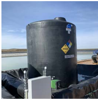
Automated Chemical Injection
