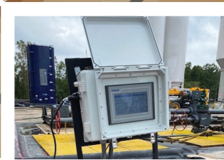
M.E.G.A. Remote Water Quality & Leak Detection
