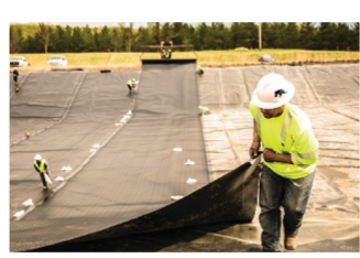
Fly Ash/Bottom Ash Storage
