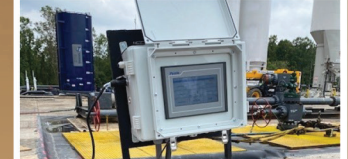
M.E.G.A. REMOTE WATER QUALITY & LEAK DETECTION
