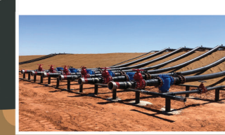
HDPE PIPE SERVICES
