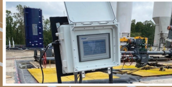
M.E.G.A. REMOTE WATER QUALITY & LEAK DETECTION
