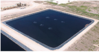
SUBSURFACE AERATION AND CHEMICAL INJECTION
