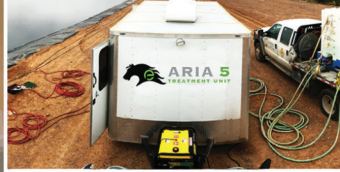
ON-THE-FLY MOBILE WATER TREATMENT
