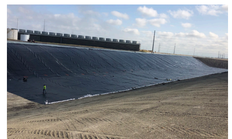
San Miguel Lignite Power Plant, Jourdanton, TX
