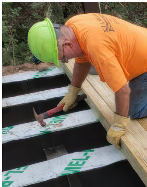
Installing clips on leading edge of first panel, after panel is slid tight to the end plate.
