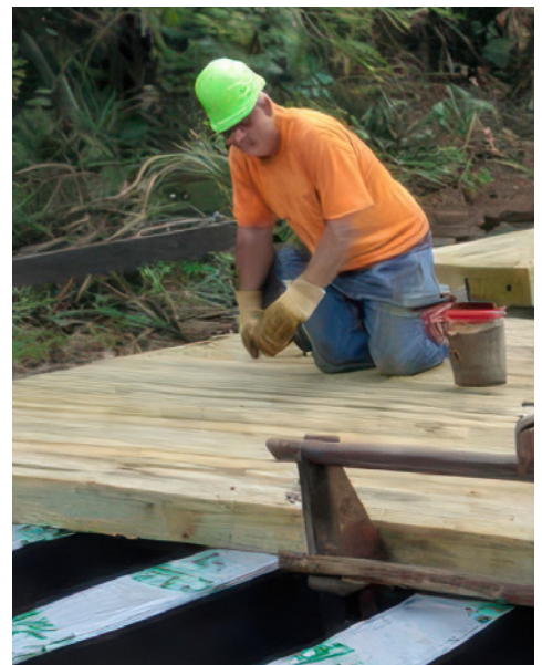
Second panel set tight to first panel with clips installed on the leading edge.
